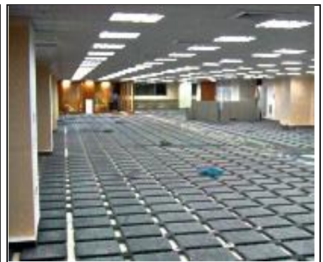
Continuous interlocking process to lay UniPanels on the floor. It follows the floor contour with no leveling needed.
